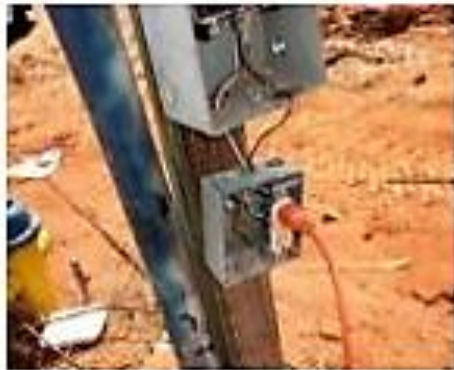
Exposed electrical parts
