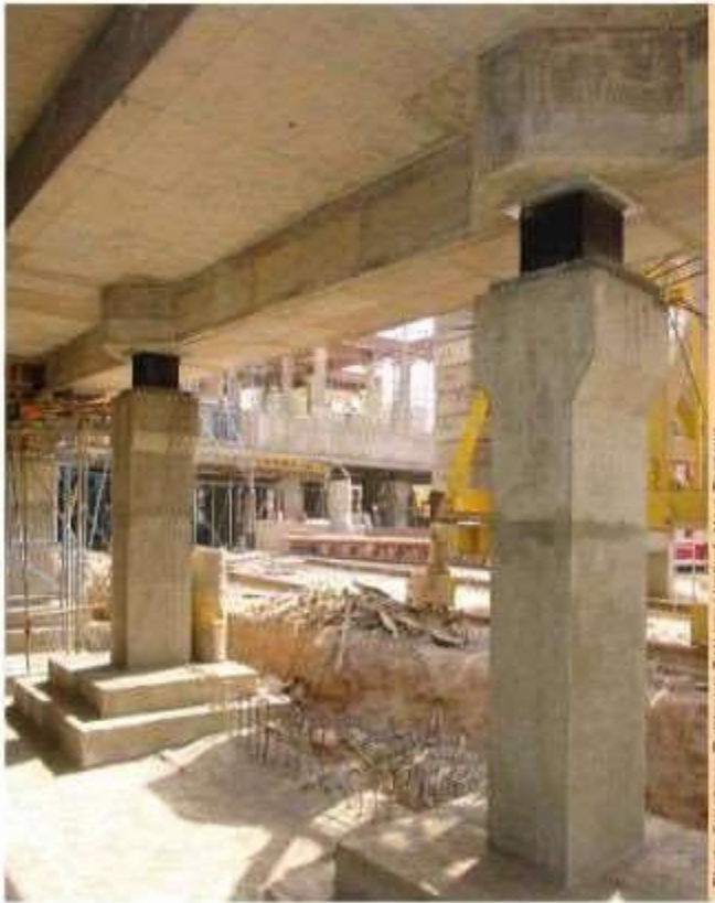
Figure 13 Piers with the lead-rubber bearings at Bhuj District Hospital
