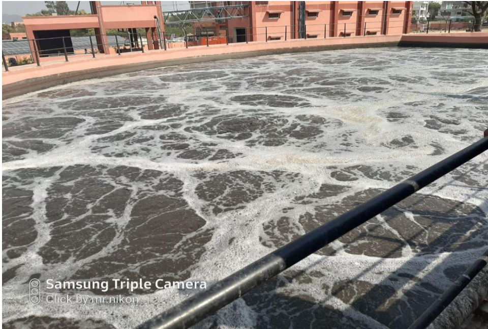
Aeration Process at the sewage treatment plant
