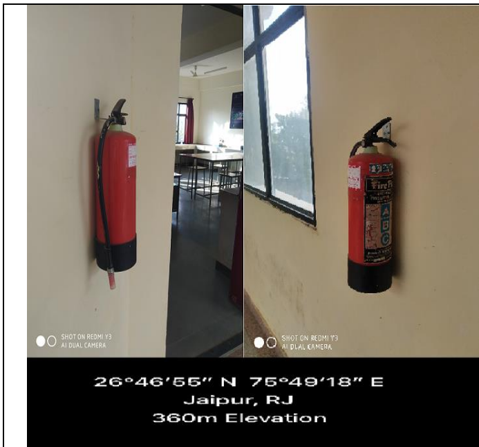
Fire Extinguisher in C-Block
