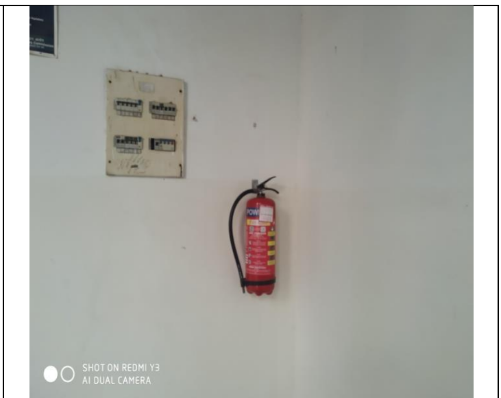
Fire Extinguisher in A-Block
