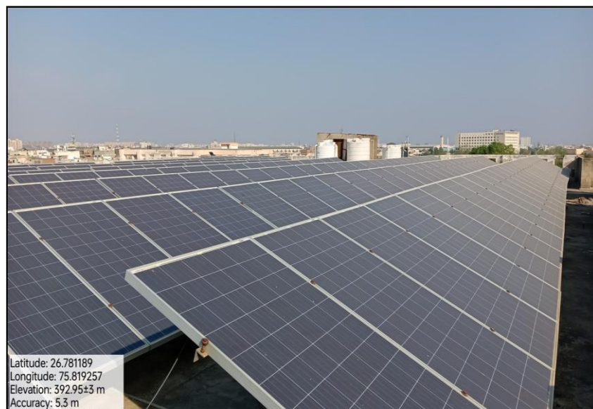
Photographs of Solar Panel
