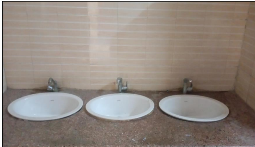
Photographs of Faucets used in Washroom
