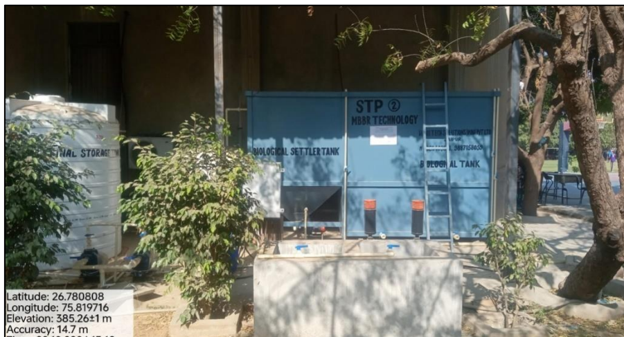
Tank for STP
