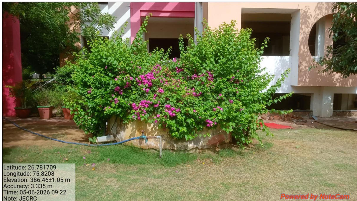
Rain Water Harvesting Tank
