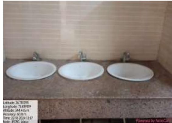
Faucets used in Washroom
