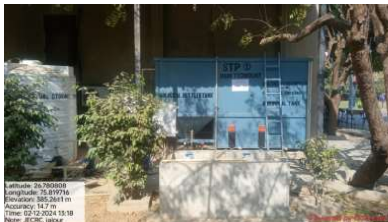
Tank for STP
