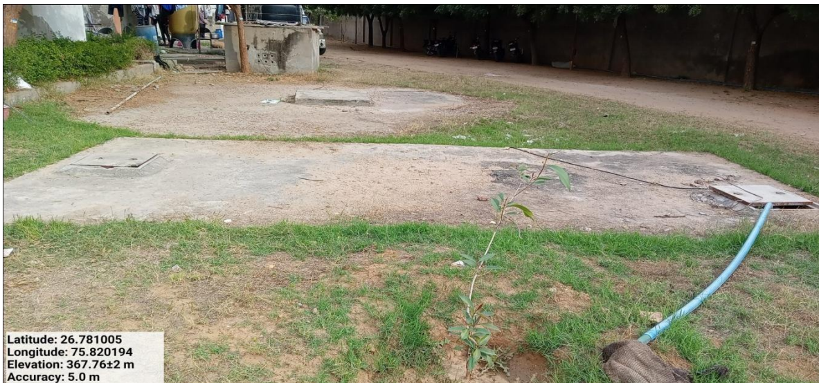
Septic Tank (Liquid Waste Management)
