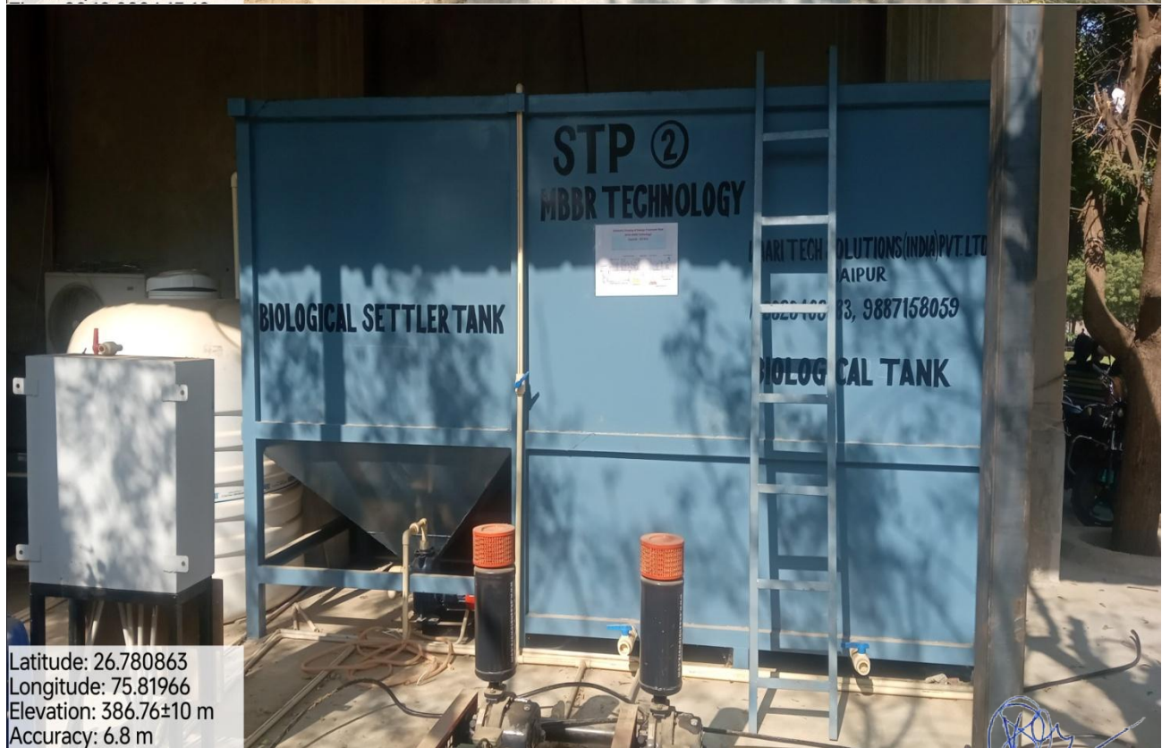
Sewage Treatment Plant
